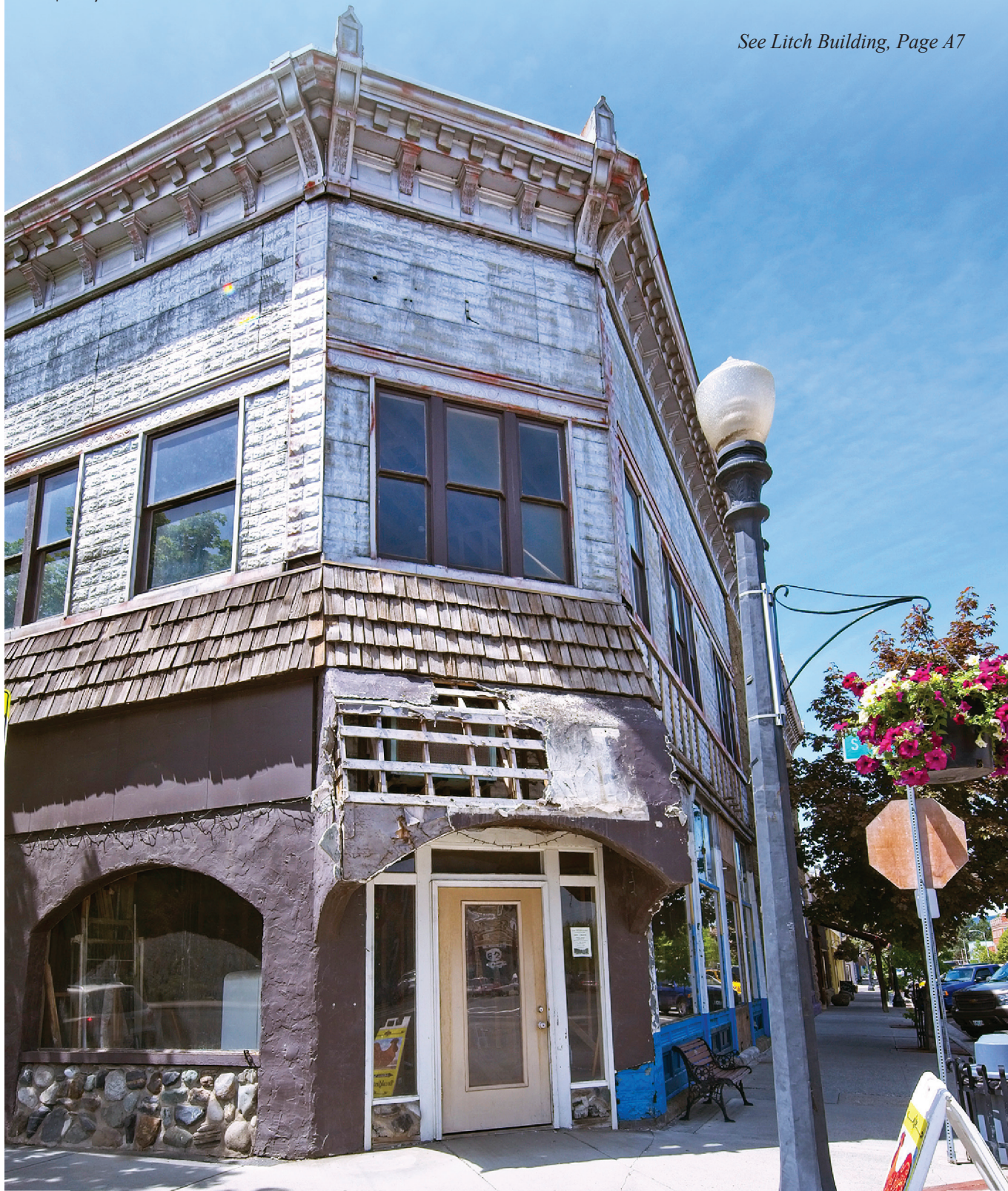
The Litch Building, at the corner of River and Main Streets in Enterprise, was built originally in 1903, and is undergoing remodeling by Andy McKee.
