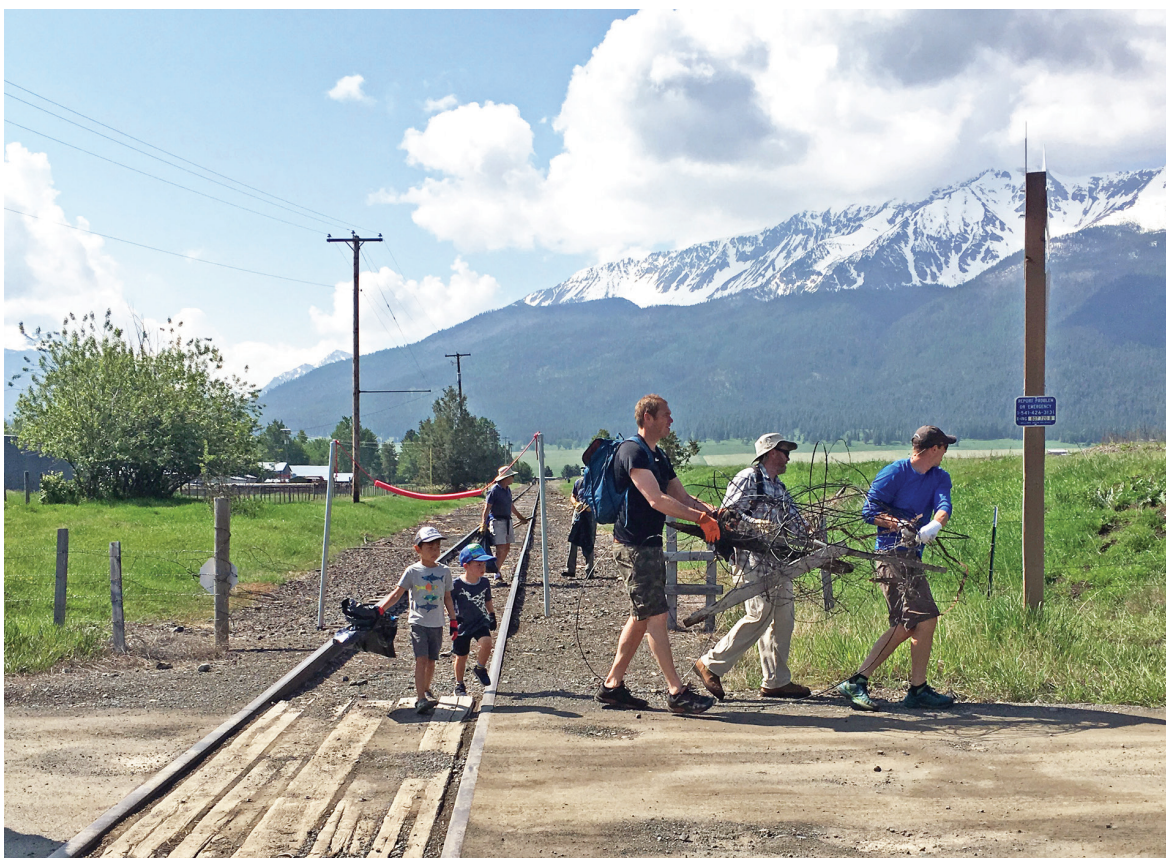
Contributed photos/Penny Arentsen Volunteers with Rails with Trails remove old fencing and other industrial debris from the railroad right-of-way during their walk on Saturday, June 1.
