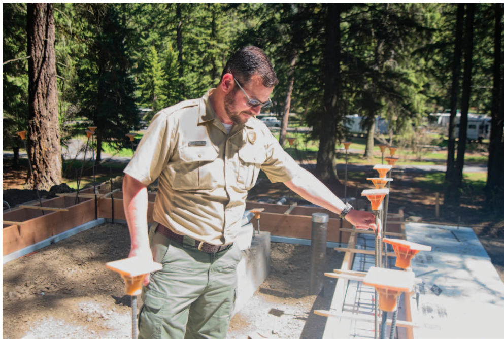
Mac Freeborn, the new manager at Wallowa Lake State Park, inspects the foundation for the park's new micro hydro power generation plant.
