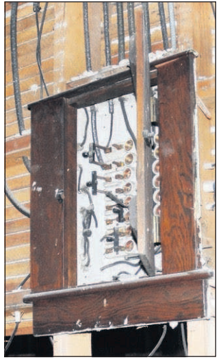
Kathleen Ellyn/Chieftain An example of the aged wiring McKee's crew had to completely tear out and replace in the Litch Building.
