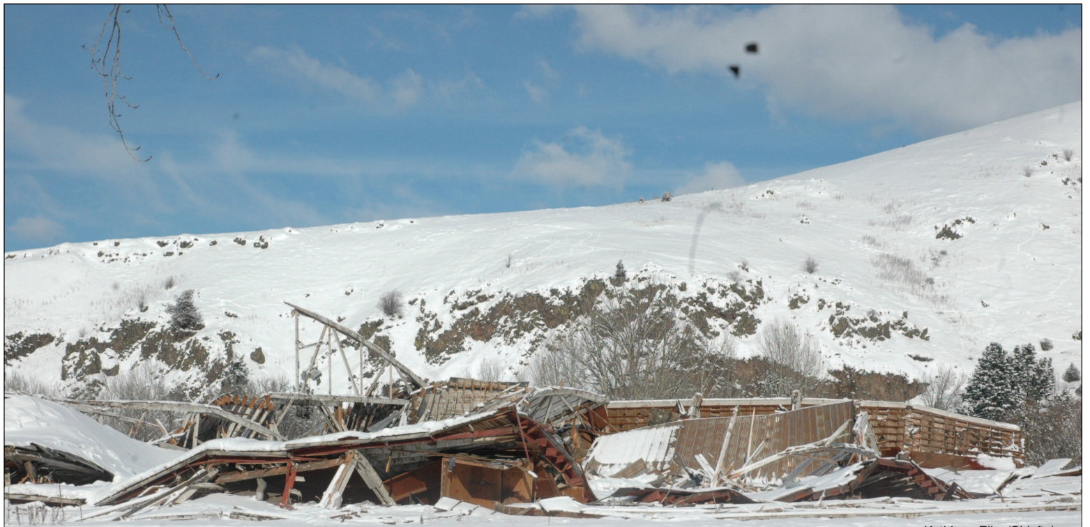
The historic J. Herbert Bate Lumber planing mill in Wallowa fell due to heavy snow.
