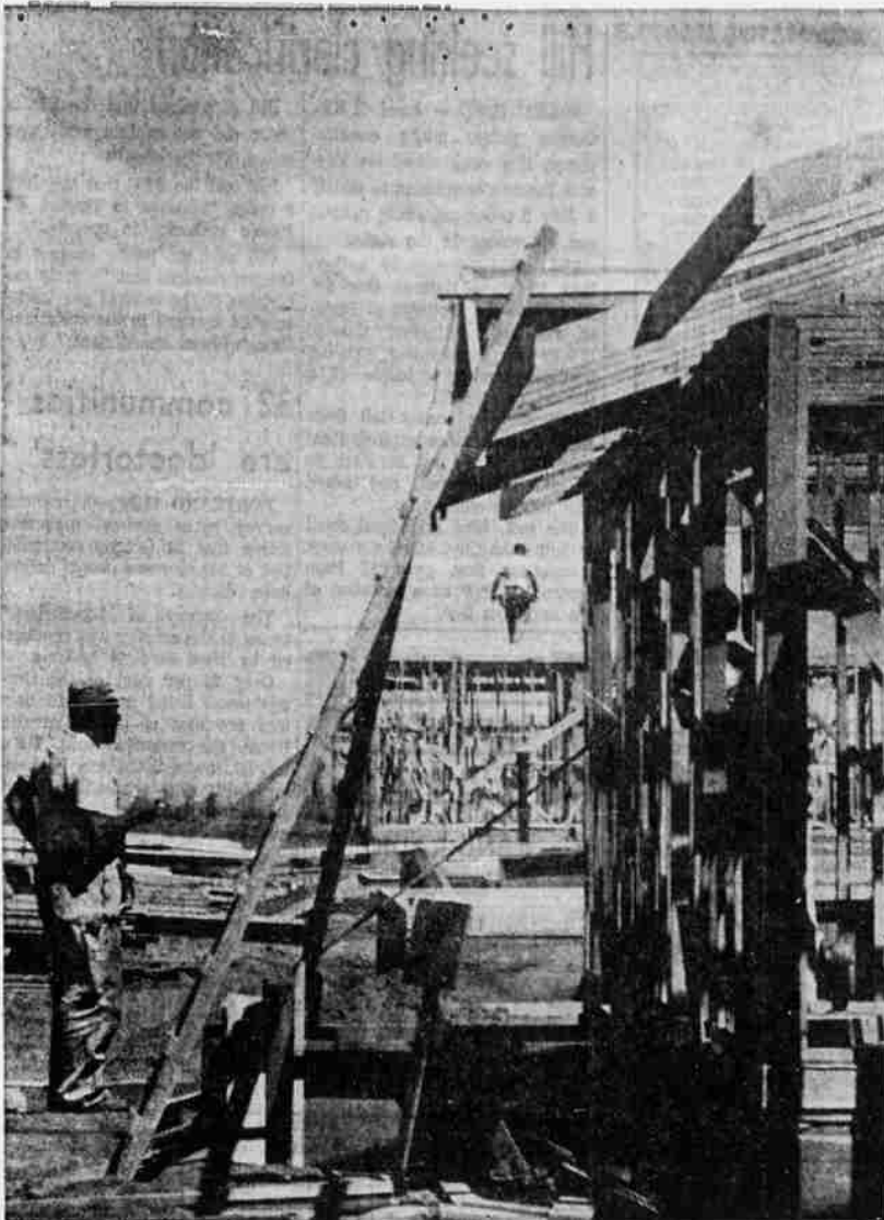
GOING UP FAST — Construction activity is booming in the new North Pilot Bridge Addition off Jones Road in Bend. Western Development Co. has 46 new homes scheduled.
