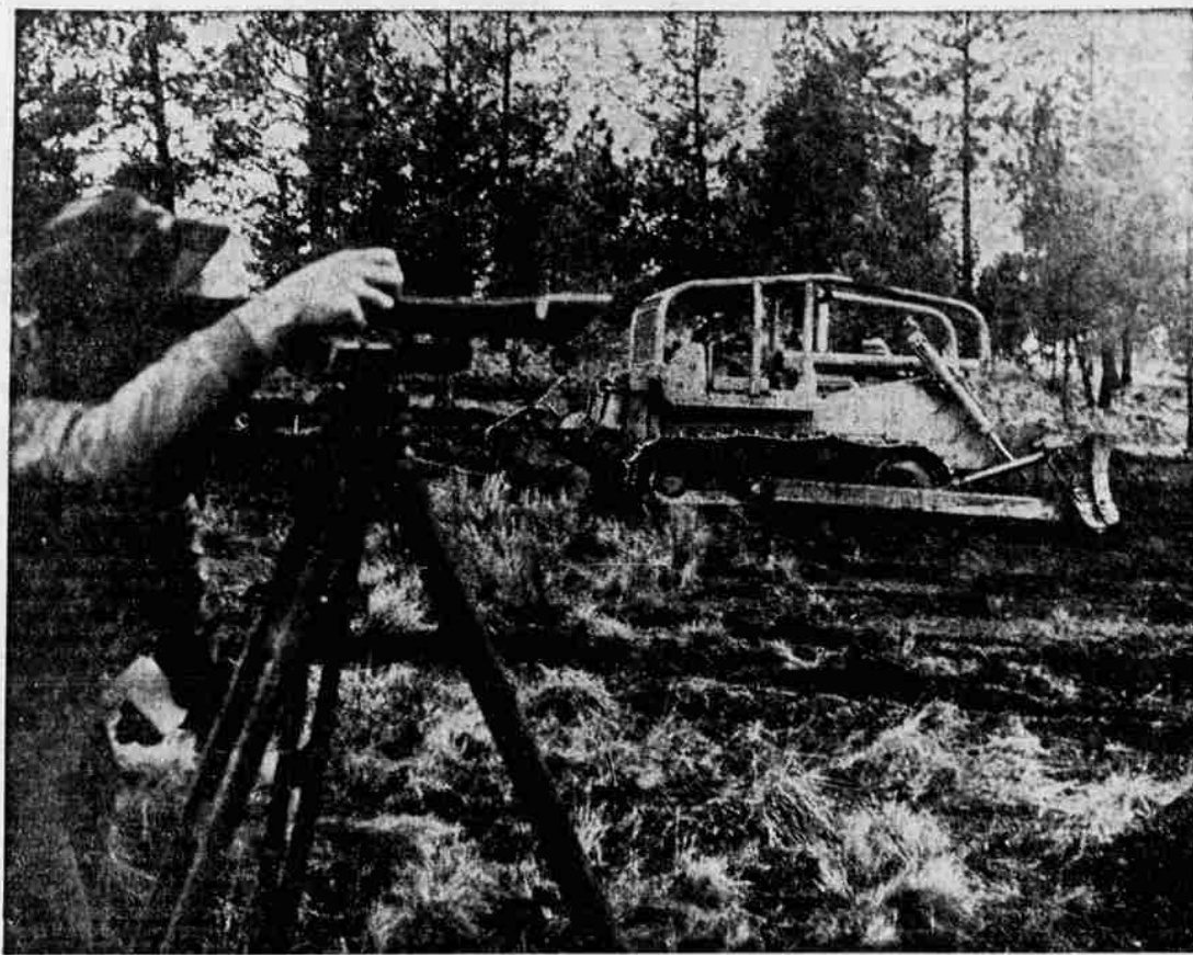
INITIAL CONSTRUCTION PHASE—The multi-purpose athletic court addition to Juniper Park planned by the Bend Rotary Club underwent its initial construction today when a bulldozer and operator were donated by Brooks-Scanlon for leveling of the court area. Glen Harvey, assistant city engineer, stands in the foreground with a survey level. The finished court will be of smooth-finish cement slab construction with lighting which will allow greater utilization of Juniper Park and more complete use of the adjacent Bend swimming pool.
