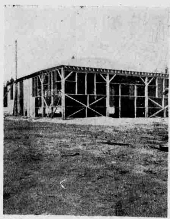
NEW BUILDING OCCUPIED — Despite the fact that it is not yet finished, the new community club building in Crescent was placed in use this week when a meeting was held. This is a view of the building, with windows still missing and some side walls to be constructed.
