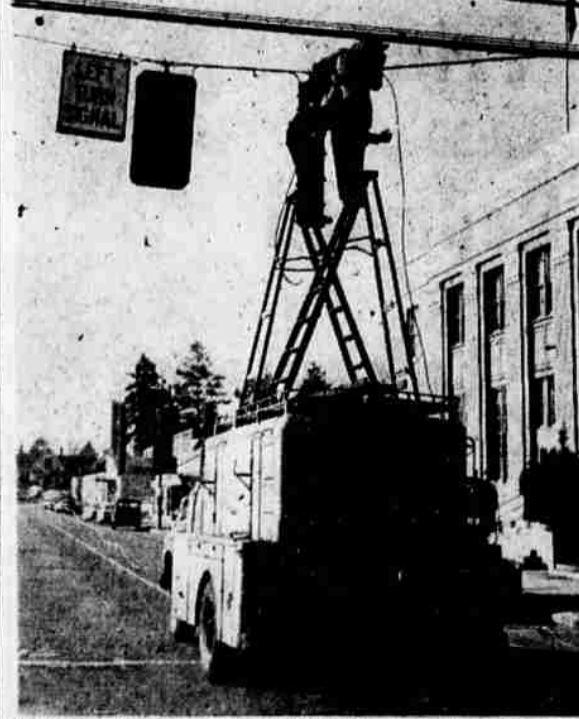
UP WITH THE NEW, DOWN WITH THE OLD—Lighting engineers from the State Highway department are shown removing the old five-lamp traffic signal that directed south bound traffic on Wall at the intersection with Franklin. To the right of the workmen is one of two substitutes for the old signal. Two new signals were installed yesterday, one controlling traffic turning left onto Franklin from Wall, shown in this picture, and one over the right lane of traffic controlling traffic moving south on Wall or turning right toward Drake Park. (Bend Bulletin Photo)
