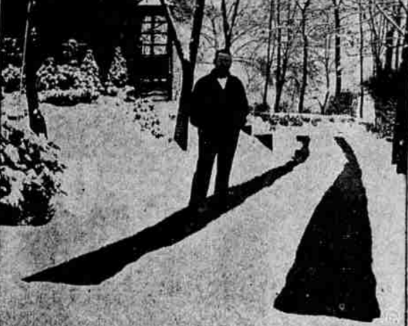
There's snow everywhere—except on those two driveway ribbons. And not an ounce removed with a shovel. Joseph C. Keane of Pittsburgh, Pa., placed a series of hot water pipes under the driveway. Results: 15 inches of snow disappeared in two hours at a cost of 60 cents for fuel. He uses an anti-freeze compound to prevent melted snow from freezing.
