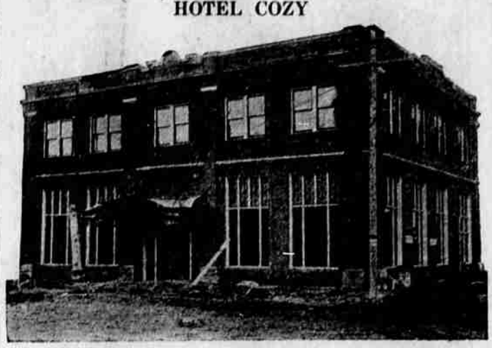
New hotel opened today by Mrs. Nettie Stevenson. —Photo taken during construction.
