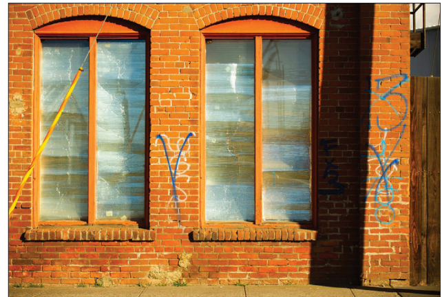
Greg Lehman/Walla Walla Union-Bulletin, File Grffiti mars a building Feb. 16, 2022, on Robbins Street in Milton-Freewater. Police reported arrested a 14-year-old on Aug. 2 in connection to 15-20 graffiti cases.
