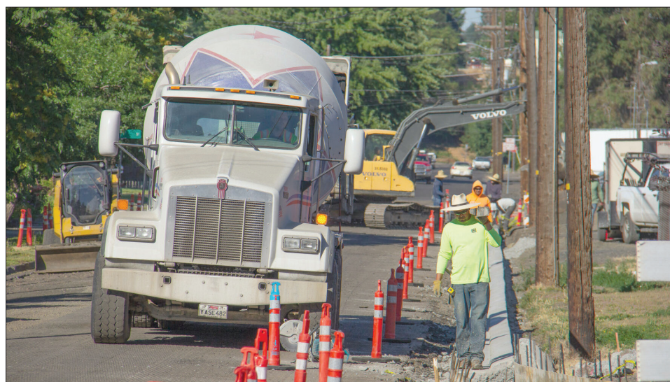
A construction crew Wednesday, July 20, 2022, works on curbs and gutters on Southeast Third Street and Goodwin Avenue in Pendleton.
