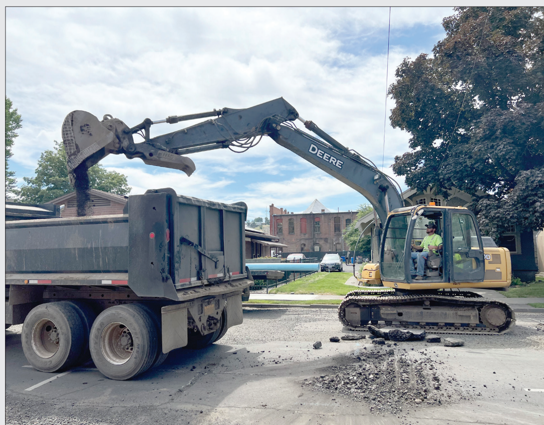
A city of Pendleton employee uses an excavator to dump gravel into a truck Thursday, June 30, 2022, while working on a construction project on Southeast Byers Avenue, Pendleton. Charly Hotchkiss/ East Oregonian
