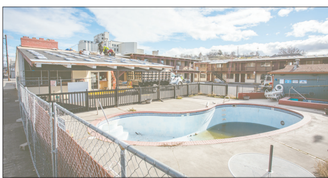
East Oregonian, File A new roof is under construction Feb. 1, 2022, at the former Knights Inn in downtown Pendleton. Portland-based Cascadia Hospitality bought the motel late last year and is on the verge of opening it as the 40-room MotoLodge. The $1.3 million renovation includes a $500,000 grant from the Pendleton Development Commission.
