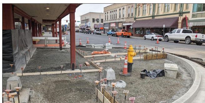
Phil Wright/East Oregonian Curb and sidewalk improvements remain underway Tuesday, April 19, 2022, along the Southeast Court Avenue side of the Hamley Western Store & Saddle Shop in downtown Pendleton.
