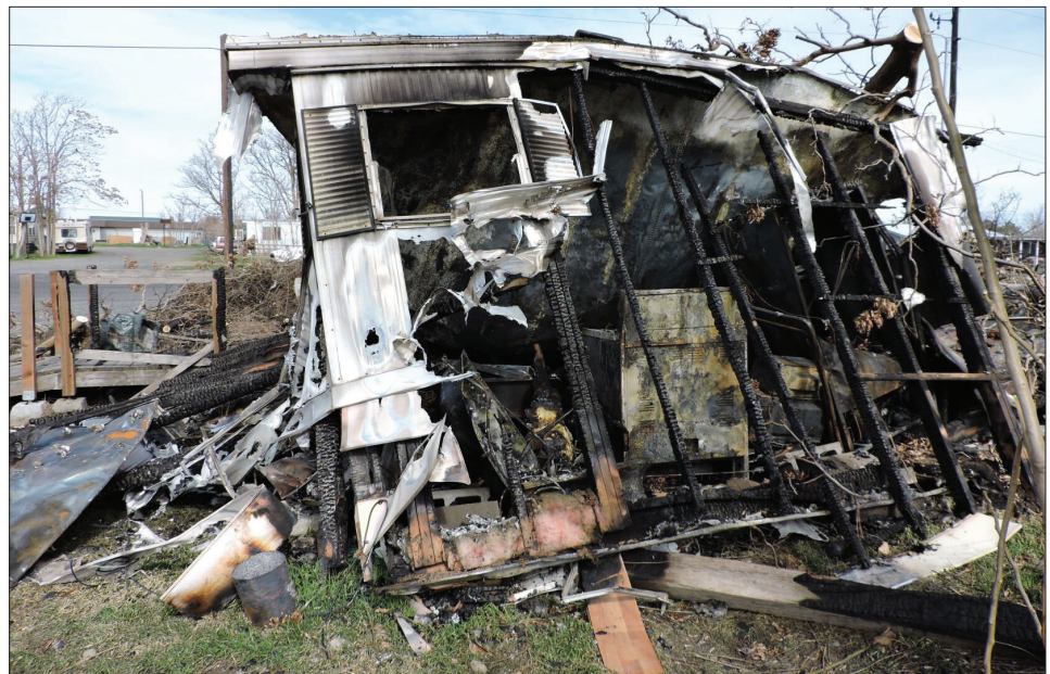
A toppled and burned mobile home sits in Irrigon on Thursday, March 10, 2022, days after a fire.
