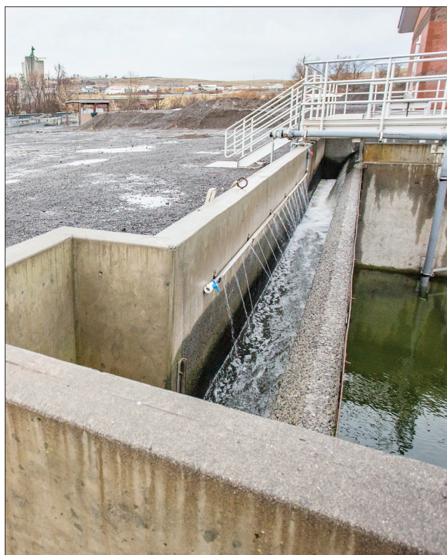
Treated water flows along a channel Dec. 19, 2019, at Pendleton’s wastewater treatment plant before being piped to the Umatilla River. The Pendleton City Council at its upcoming meeting on April 5, 2022, could vote on increasing city utility rates.
