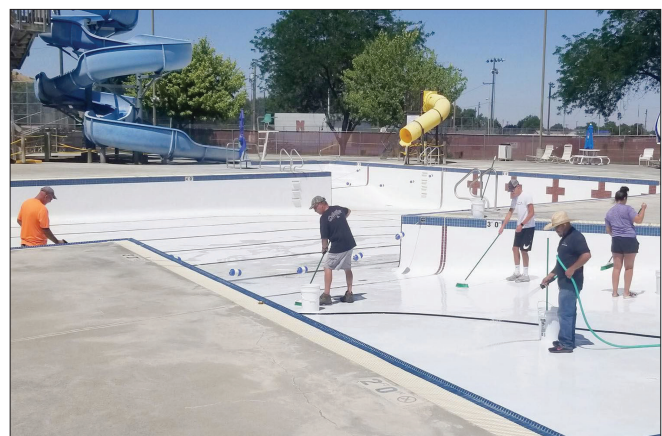
City crews scrubbed surfaces of the Milton-Freewater public pool in 2019 to remove a failed coating product.
