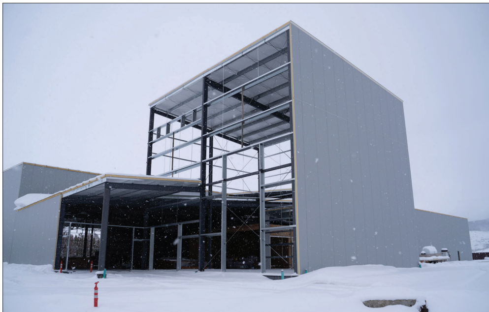
Snow accumulates on the nearly finished frame of the Eastern Oregon University fieldhouse on Tuesday, Jan. 4, 2022.
