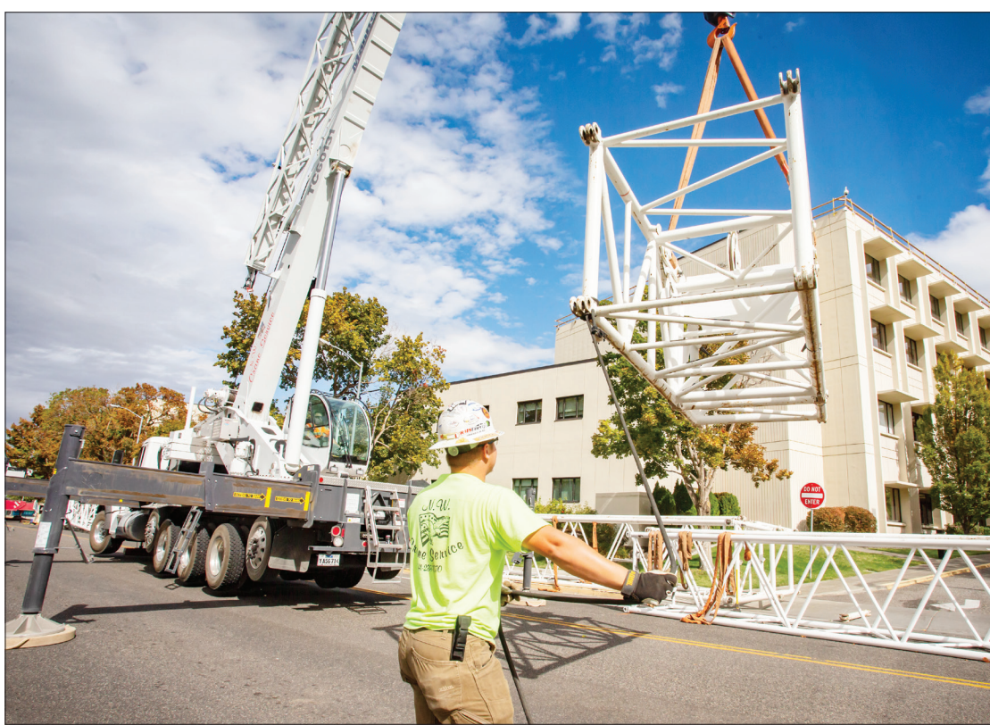
Ilyas Harral, of Pendleton, uses a rope to guide a crane segment into position Monday, Sept. 27, 2021, while working with Hermiston-based N.W. Crane Service Inc. at Kadlec Regional Medical Center in Richland, Washington.
