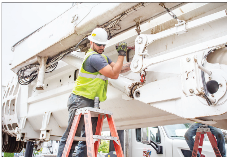
Riley Sederburg, of Adams, lines up a hydraulic component while working with Hermiston-based N.W. Crane Service Inc. to assemble a crane Monday, Sept. 27, 2021, at Kadlec Regional Medical Center in Richland, Washington.
