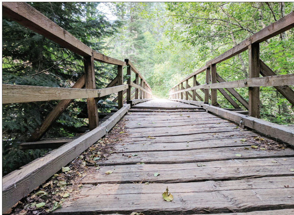
U.S. Forest Service staff in 2013 discovered the Burnt Cabin Creek Trail Bridge was deteriorating in the Umatilla National Forest's Walla Walla Ranger District. The forest is receiving funds to replace the bridge.
