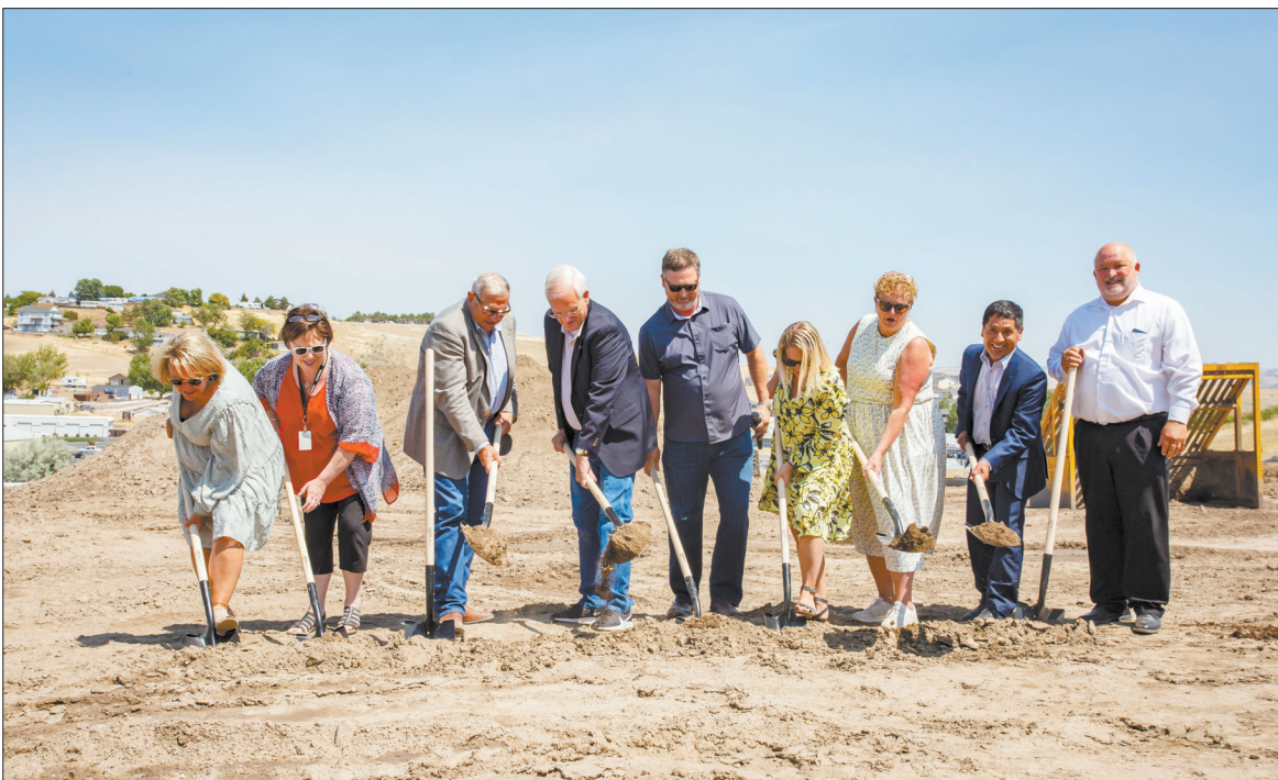
A group of local officials and stakeholders break ground Wednesday, July 21, 2021, on the 80-unit Wildflower Apartments affordable housing complex in Pendleton.
