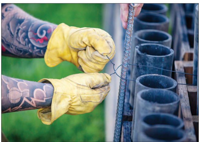
Mark Pursel ties wire around pieces of rebar Sunday, July 4, 2021, to support the fireworks launchers in preparation for the annual Stanfield Fourth of July fireworks show.
