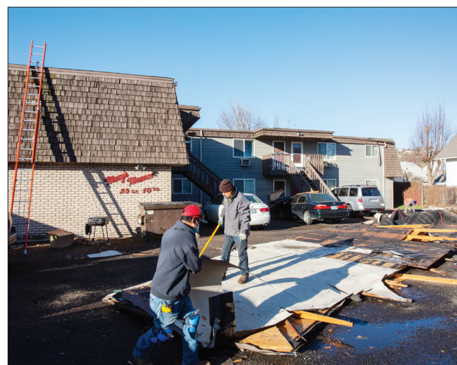
Construction crews work to dismantle the destroyed roof of Mary's Mannor after it was blown from the building on Wednesday, Jan. 13, 2021.
