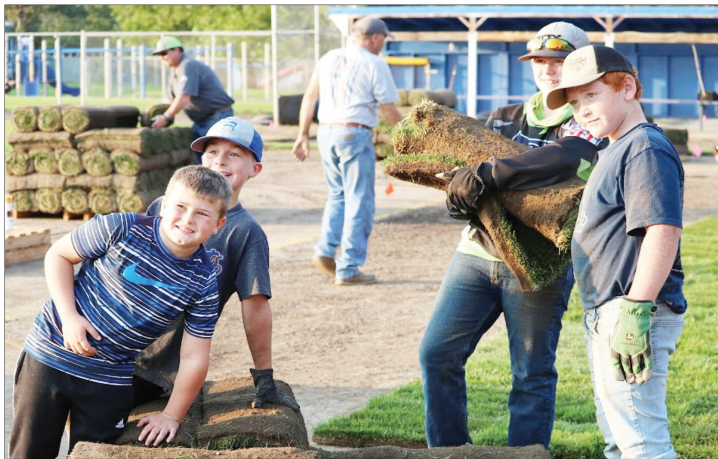
A group of boys help lay sod during a work party to repair the damaged Pilot Rock Little League field on Sept. 30, 2020. The ball field was damaged by a flood on May 20, 2020, when East Birch Creek burst its banks and flooded the field and other portions of Pilot Rock.
