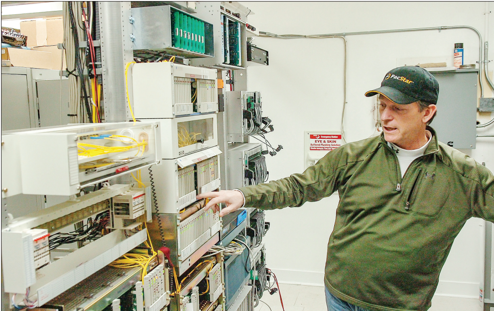
Former Helix Telephone Company co-owner Jim Smith gestures toward equipment while explaining how the telephone exchange works in the Helix Telephone Company central office in Helix on Feb. 14, 2012.
