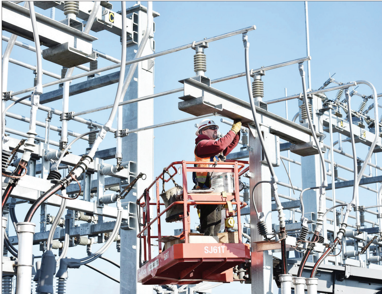
A substation technician installs a ground wire on a riser structure in December 2017 at a new Umatilla Electric Cooperative substation on East Elm Avenue in Hermiston. EO file photo
