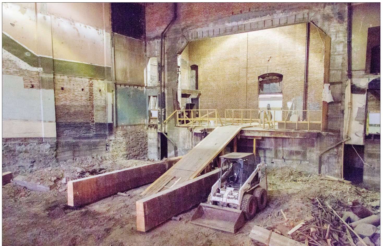
Staff photo by Kathy Aney A large beam that once spanned the width of the Rivoli sits in pieces on the historic theater's dirt floor during Saturday's open house and workday.
