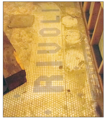
Staff photo by Kathy Aney The foyer to the historic Rivoli features the theater's name in tile. The tile will be incorporated into the new foyer.
