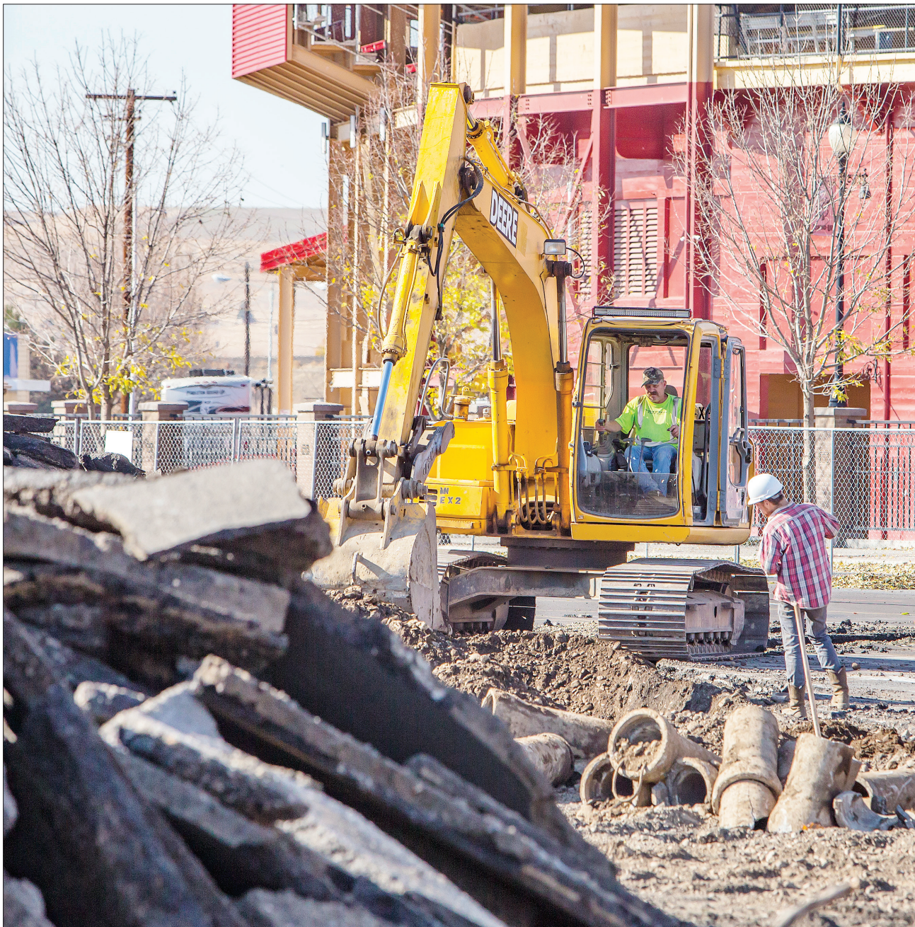
Workers tear up the asphalt parking lot at the former Albertsons site in Pendleton on Tuesday afternoon in preparation for the construction of the Pendleton Round-Up's new multi-use building at the site.
