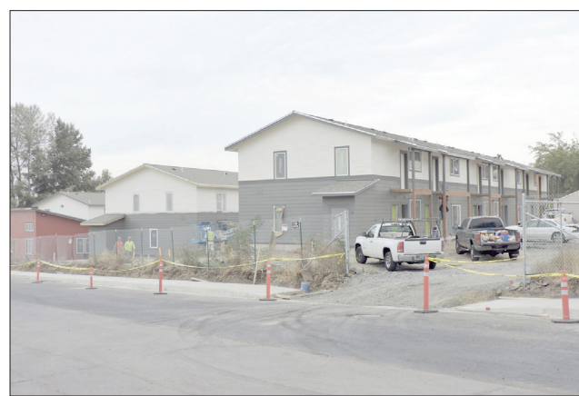
Staff photo by Jade McDowell Subsidized housing is under construction on Southeast Fifth Street in Hermiston. Most tax incentives for housing are for low-income options.
