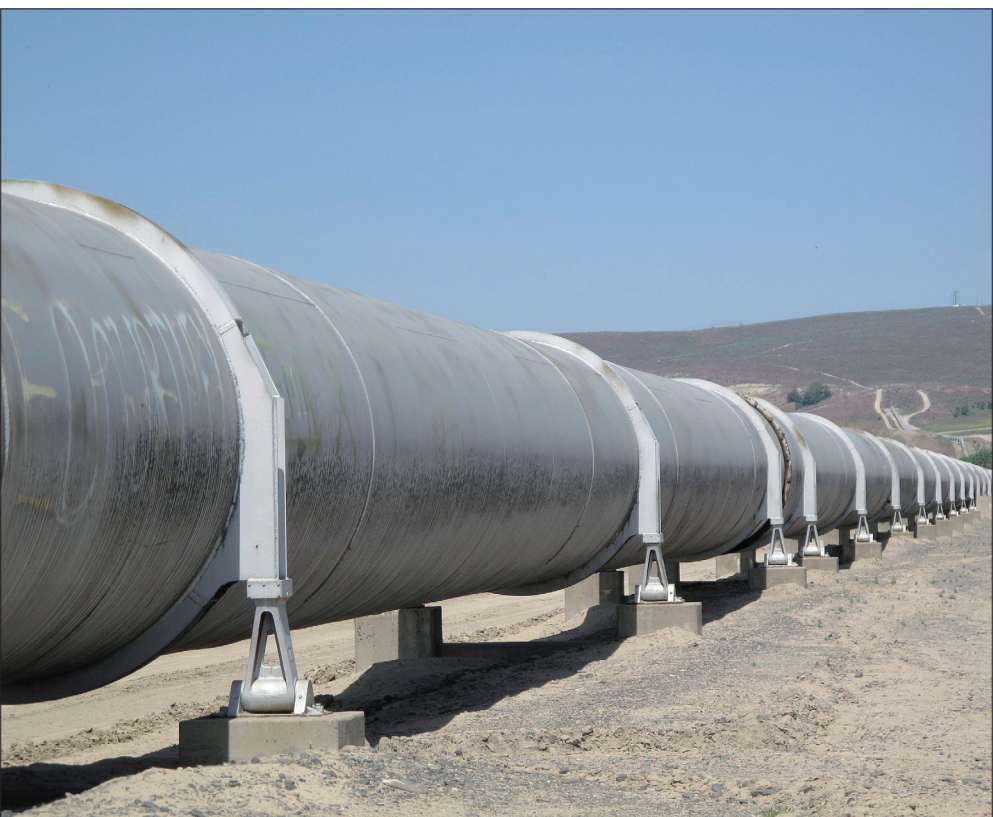
The Malheur Siphon is a 4.5-mile-long steel pipe that carries irrigation water from Malheur Reservoir to the northern part of the Owyhee Irrigation District system.
