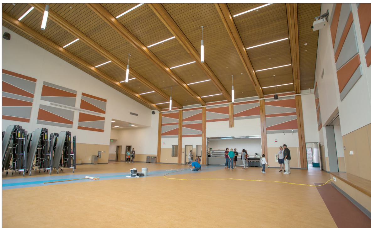
Crews work to finish the floors at the new Nixyaawii Community School during an open house on Thursday afternoon.
