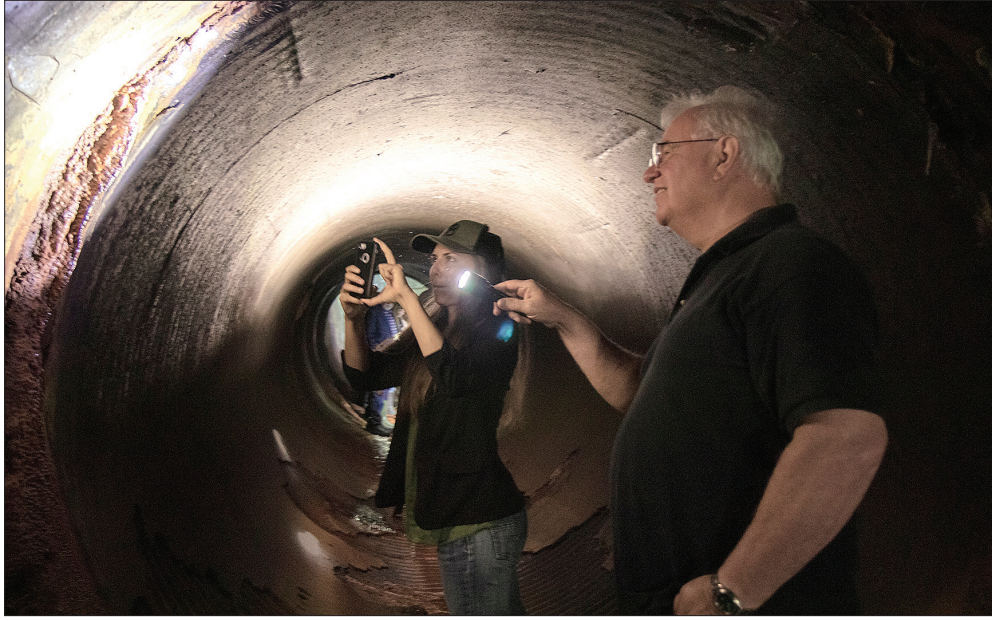
Racquel Rancier of the Oregon Water Resources Department, left, takes a photo of a seepage hole inside the Big Creek dam intake while Rep. David Gomberg, D-Neotsu, right, shines his flashlight on the vulnerable area.
