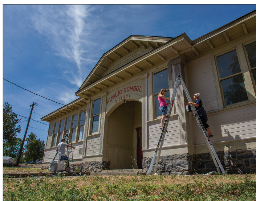
Staff photo by Ben Lonergan A fresh coat of paint is applied to the old Pilot Rock Public School building on Highway 395 in Pilot Rock.
