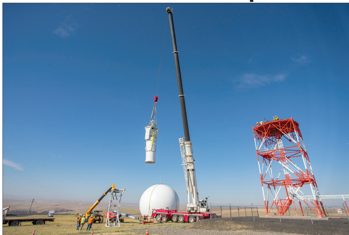
Staff photo by Ben Lonergan Crews work to lower the internal structure of the National Weather Service Pendleton radar dome Friday morning. The removal of the dome was a part of the endeavor to update and replace the radar system. The renovated radar system is expected to provide reliable data for the next 10 years, according to the National Weather Service.
