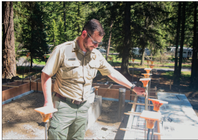
Wallowa County Chieftain Photo/Ellen M. Bishop Mac Freeborn, the new manager at Wallowa Lake State Park, inspects the foundation for the park's new micro hydro power generation plant.
