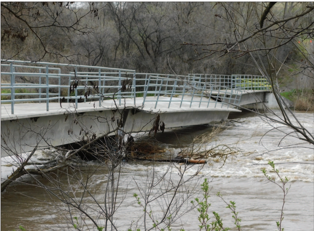
A portion of the pedestrian bridge over the Umatilla River near Umatilla High School collapsed Sunday.
