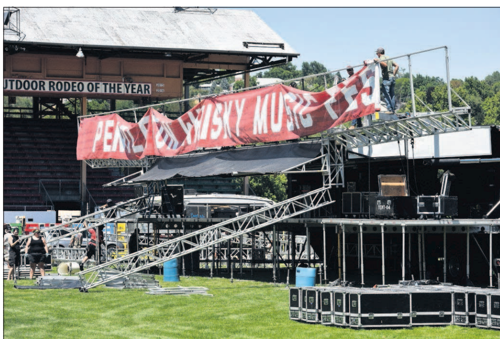
A work crew hangs a banner on the stage while preparing for the Pendleton Whisky Music Fest on Thursday in Pendleton.
