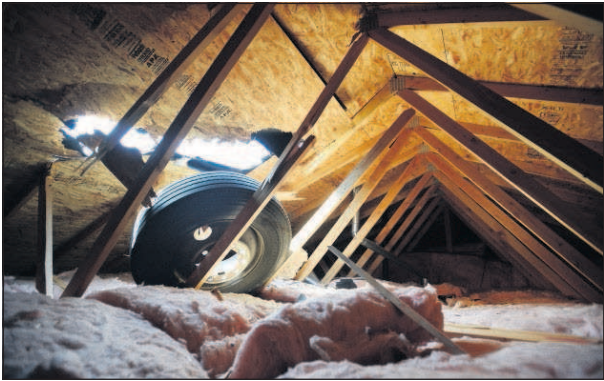
A tire and wheel sits in the attic at 114 South-west Kirk Avenue on Monday in Pendleton. The wheel came crashing through the ceiling.
