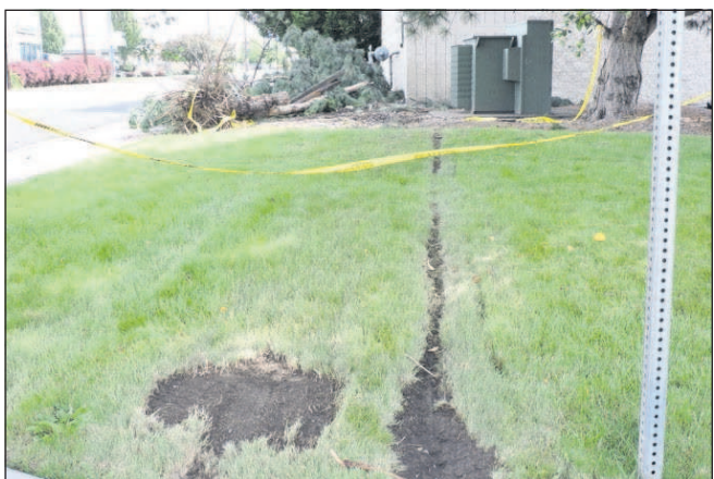
The scene behind the Pendleton Safeway shows plenty of damage from where a car crashed early Wednesday. Three passengers went to St. Anthony Hospital, a fourth received medical attention at the scene, and the driver ran but later turned himself in. Pendleton Police Chief Stuart Roberts said speed was a factor and alcohol may have contributed to the crash.
