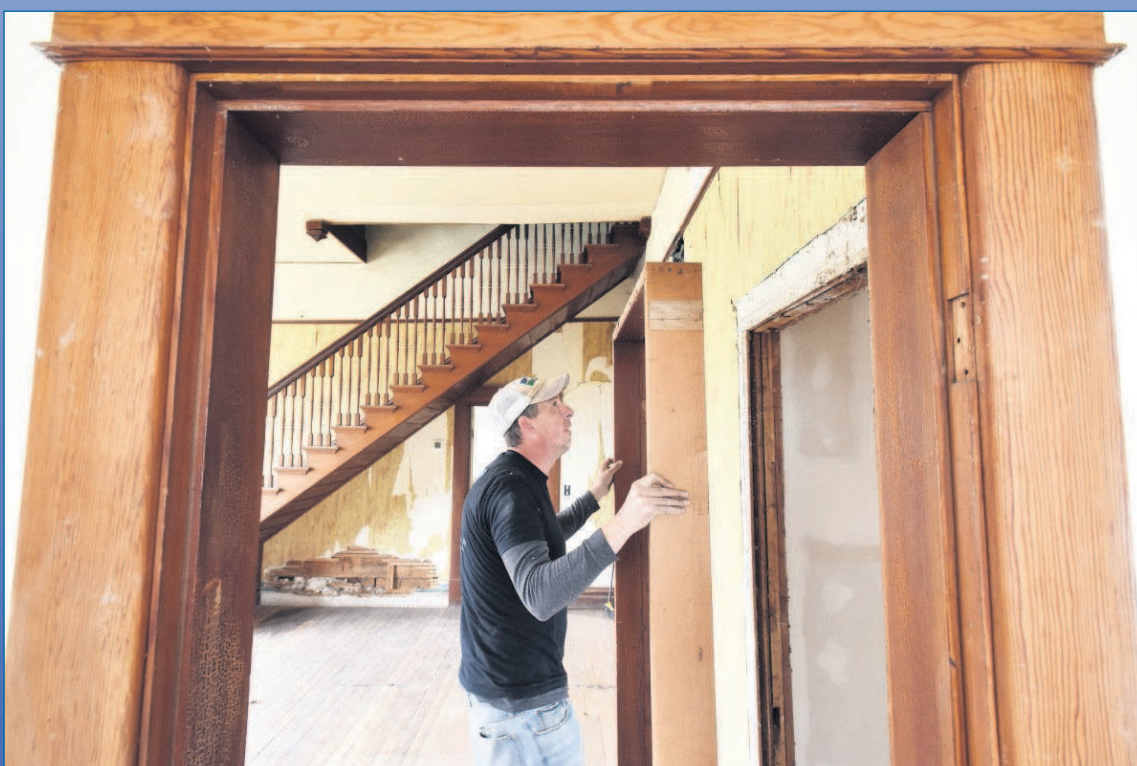
Owner-contractor Brent Webb removes a door frame while renovating his 120-year-old house on Wednesday in Pendleton. Staff photo by E.J. Harris
