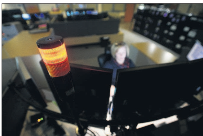
A light tower tells other dispatchers and managers whether a dispatcher is on a call or talking over the radio.
