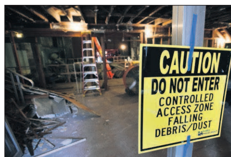
The demolition at the Rivoli Theater is 70 percent done with the goal for a completion date of April 15.
