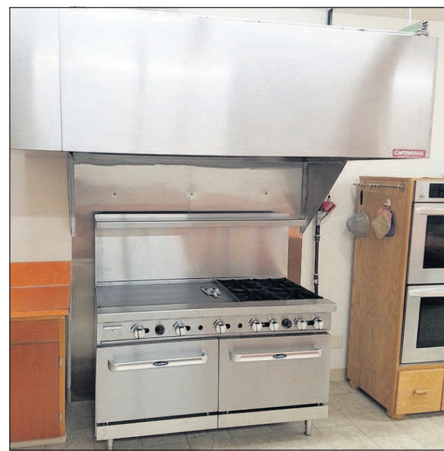
The kitchen at the Stanfield Community Center received a recent upgrade thanks to grants from the Oregon Community Foundation and Union Pacific.
