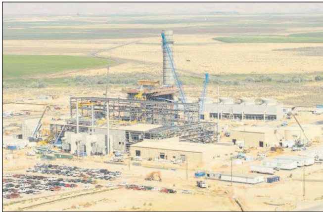
Contributed photo by Michael Durham Construction of the Carty Generating Station as seen in August 2015.
