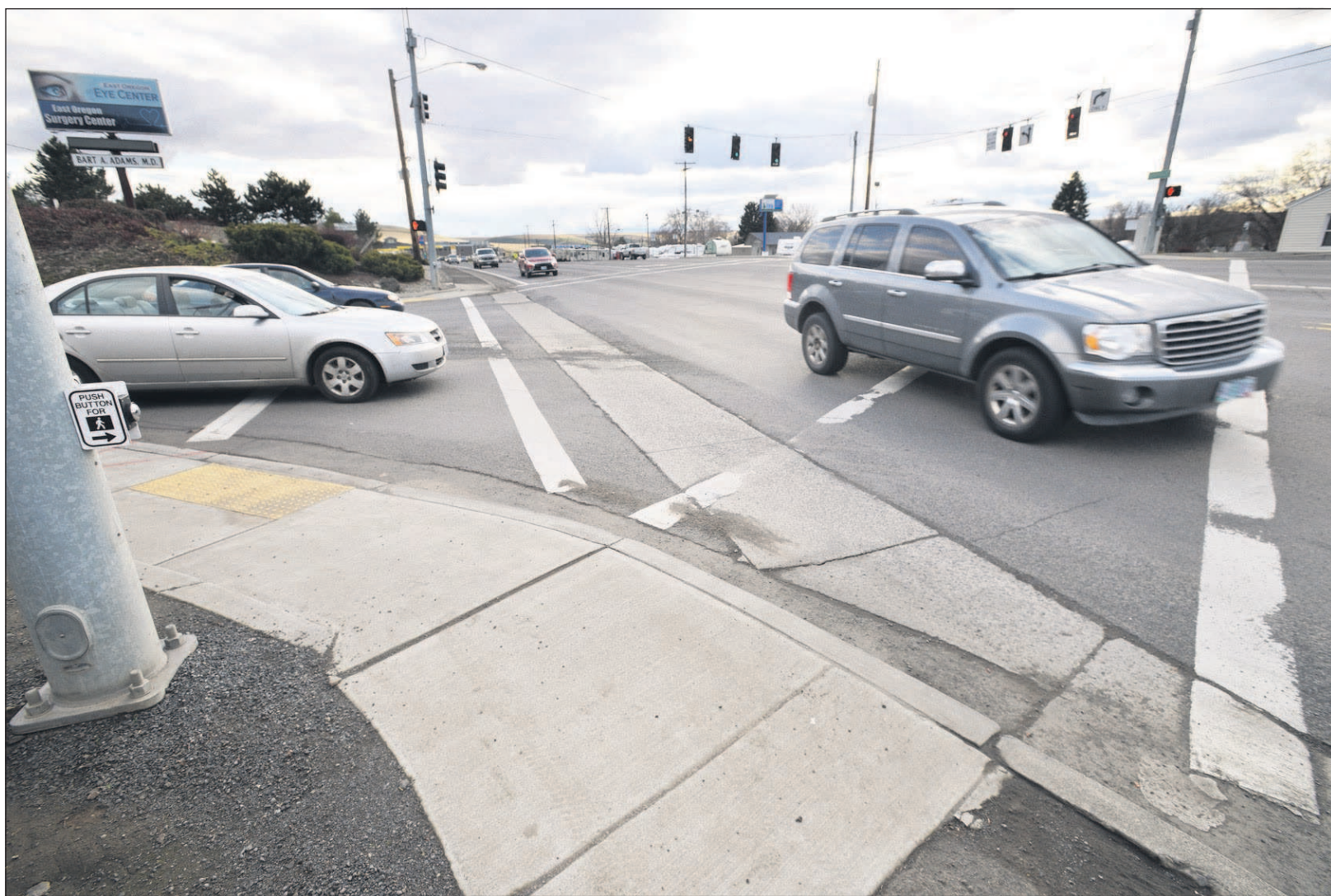
A missing wheelchair ramp at the intersection of Highway 395 and Southwest 30th Street in Pendleton would force a wheelchair user to go out onto the roadway in order to use the crosswalk that traverses the highway. A recent Oregon Department of Transportation audit found that ninety-seven percent of the curb ramps on state highways were not compliant with the Americans with Disabilities Act.
