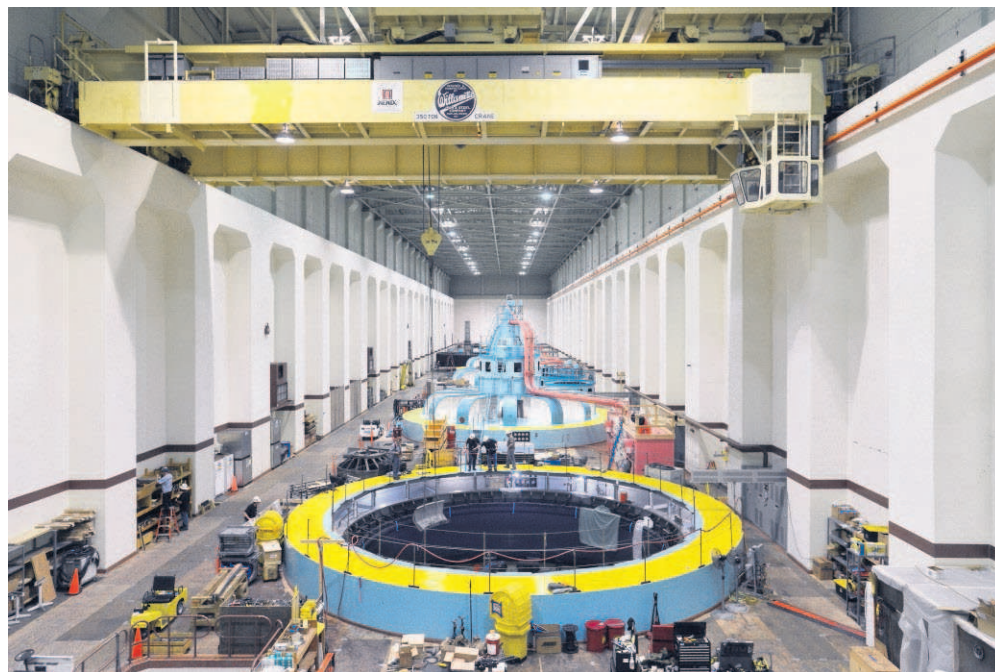
EO file photo An overhead crane is used to remove a piece of main unit power generator in 2014, at the McNary Dam on the Columbia River outside of Umatilla.
