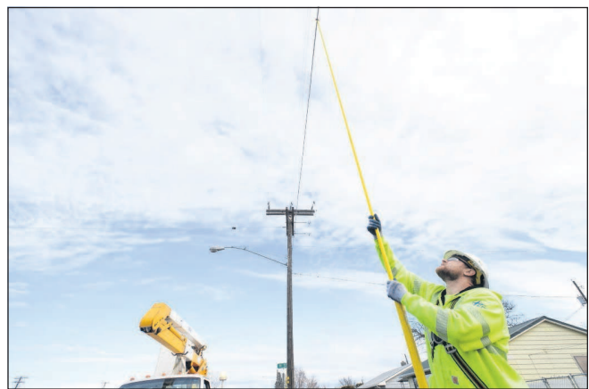
Lineman C.J. Christensen with Eastern Oregon Telecom measures the height of an internet cable line on Wednesday in Umatilla.
