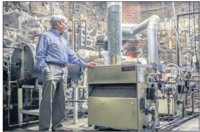
Harold Nelson, a member of the Pendleton United Methodist Church, looks after the church's boiler and does other maintenance around the building.
